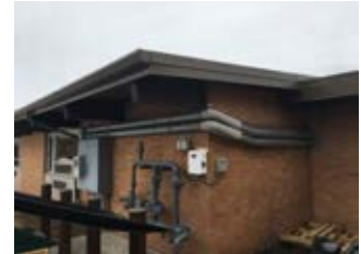
Main Electric Service Entrance
