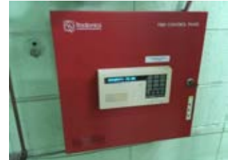
Boiler Monitoring System
