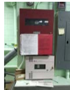
Fire Alarm Control Panel
