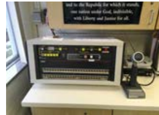
Intercom System Head-End
